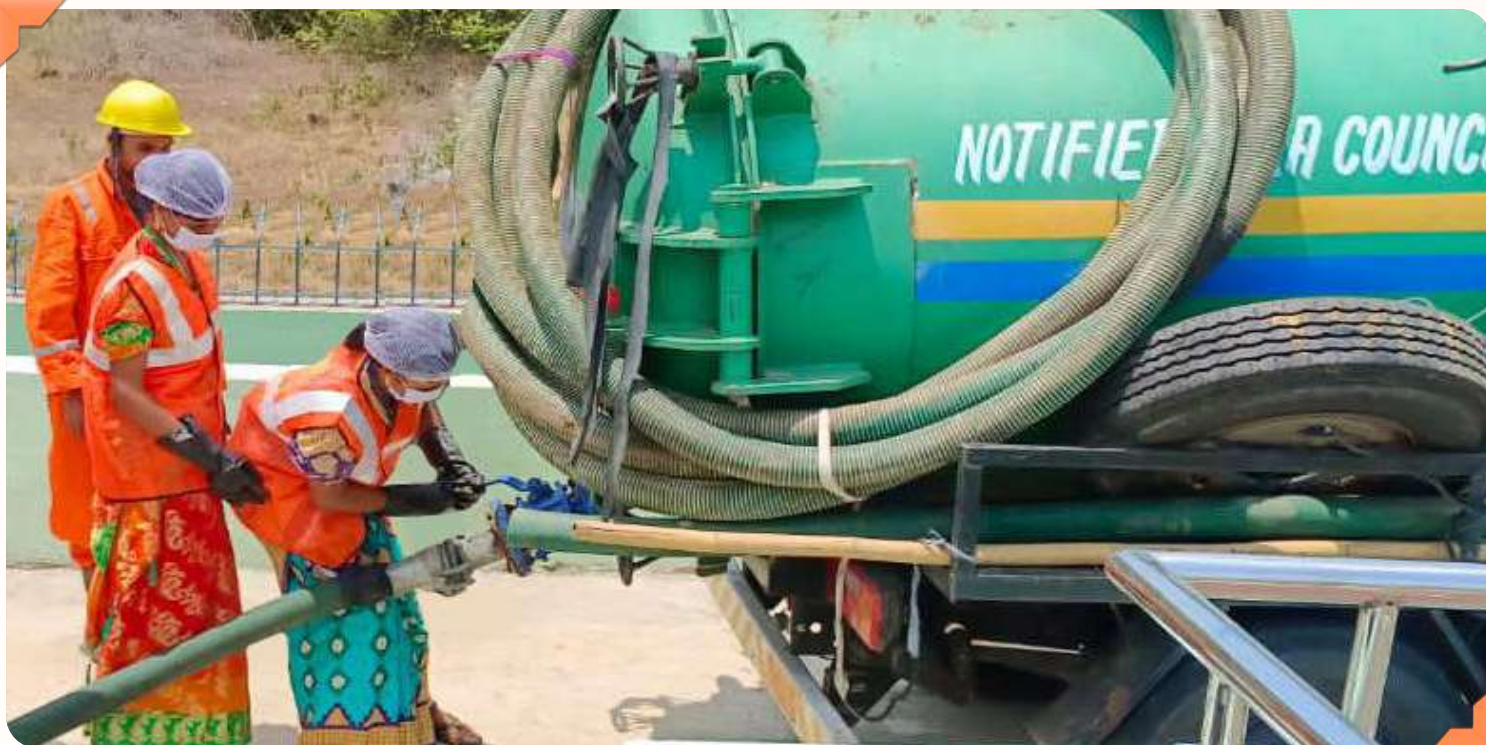
Women in Sanitation – Self-Help Groups leading cesspool maintenance efforts.
