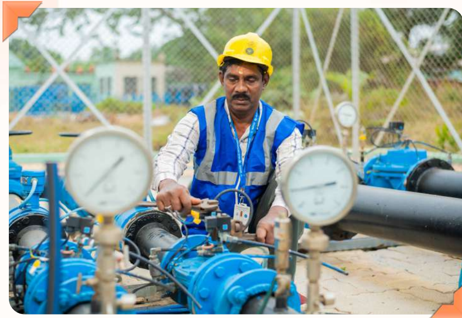
24x7 Drink from Tap – Ensuring round-the-clock safe drinking water supply through regular maintenance.
