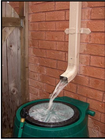
Figure. 4 Rainwater collection (through downpipes and sieves)
